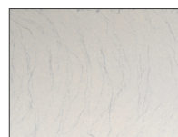
COVERAGE TOO LIGHT
